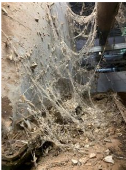
Top of Air Handling Units
