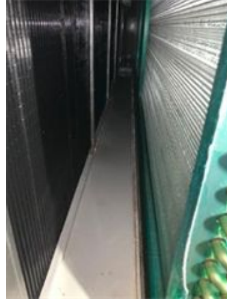
Internal AHU filters, post-clean
