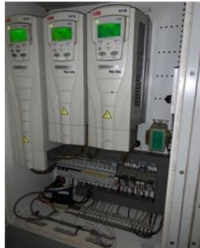
AHU control board after cleaning
