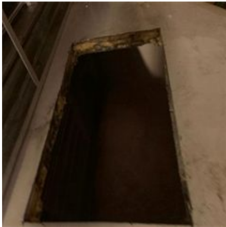
AHU duct opening pre-clean
