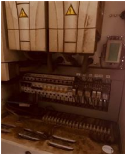
AHU control board before cleaning
