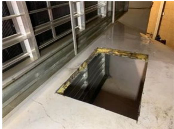
AHU duct opening post-clean
