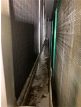
Internal AHU filters, pre-clean
