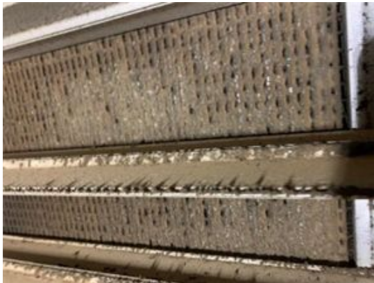
Internal AHU filters, pre-clean
